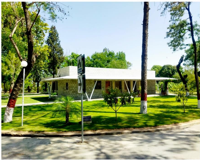
Fixing of Concrete Tiles on the External Wall of DG Camp Office
